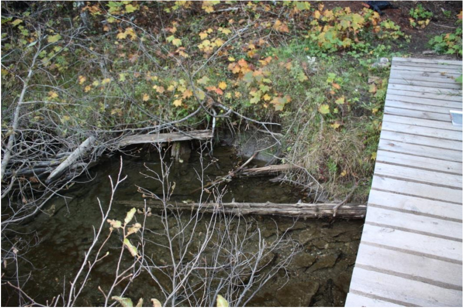
2 Photos of currently stable banks on west side of Reinecker Creek crossing
